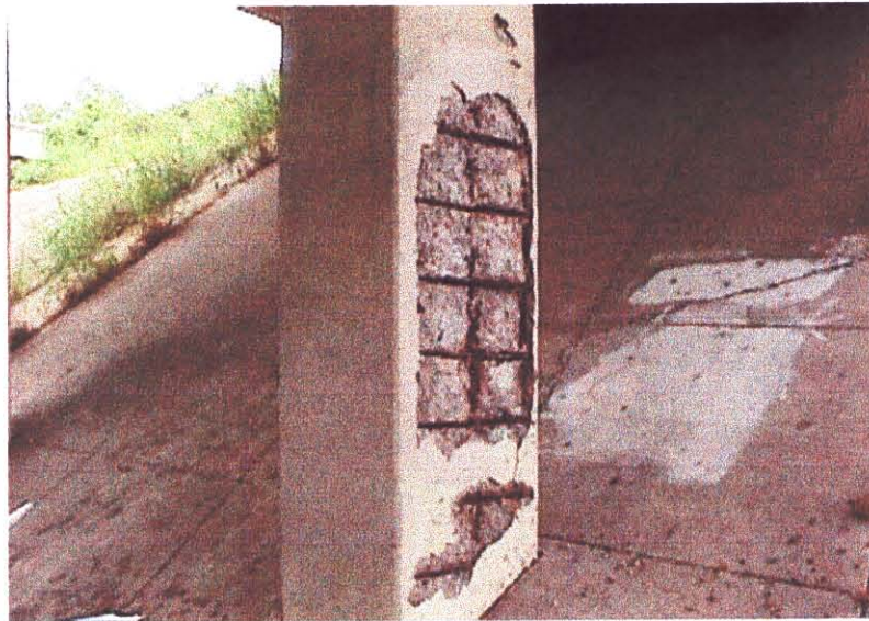
SPALL/REBAR IN COLUMN "B", BENT #3
